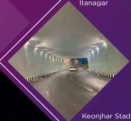
Tunnel lighting, Itanagar
