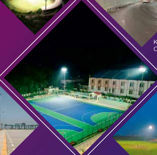
Highmast at Port
